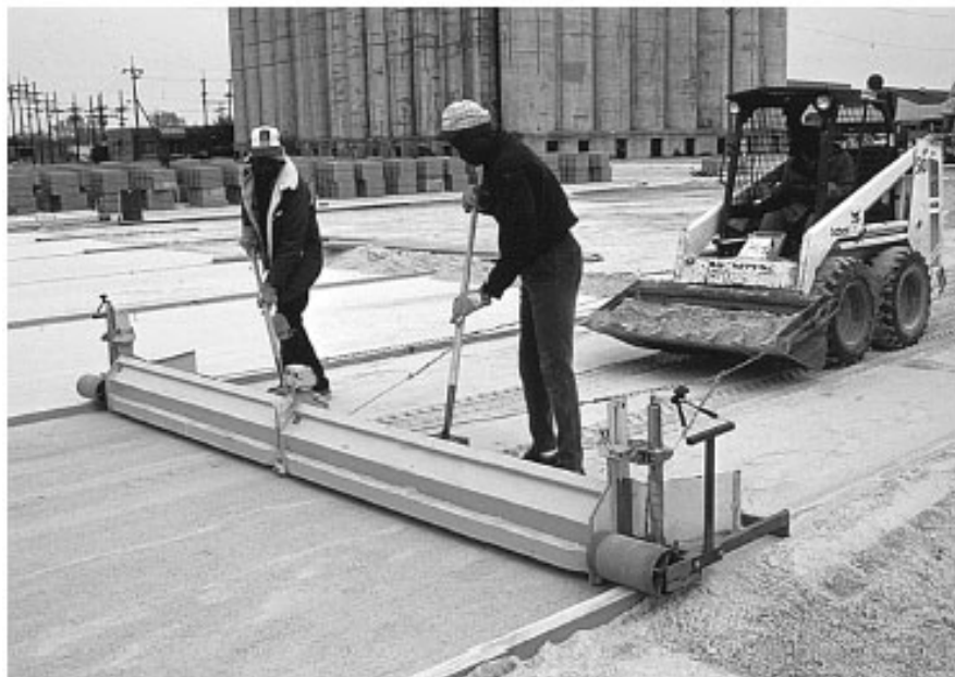
Figure 17. Powered screed bucket accelerates spreading of bedding sand. The width of the bucket can be adjusted.
